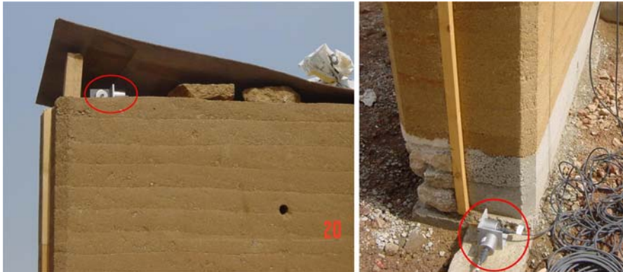
Fig. 11 Sensors disposition on top (left) and on base (right) of the wall for acceleration measurement
